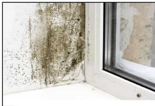
Figure 24: Mold or black spots in wall to be cleaned with bleach
